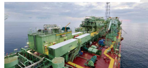
△ Offshore production facility
