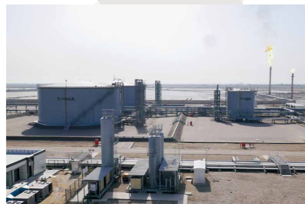
△ Central production facility
