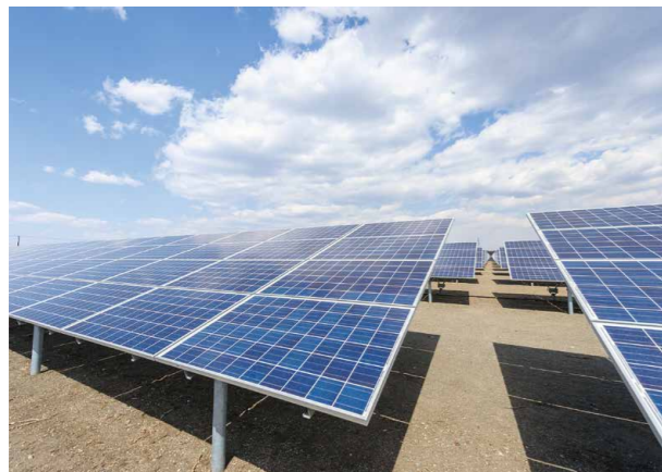
△ Our mega-solar power plant in Hokkaido
