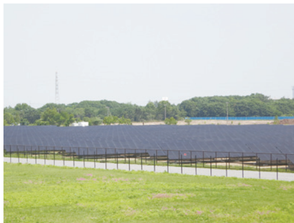
Mega-solar power plant at the Hokkaido District Office
