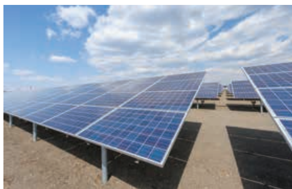
Solar panels (Solar Power Tomakomai Co., Ltd.)
