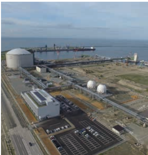
Panoramic view of the Soma LNG Terminal construction site (Soma Port, Fukushima Prefecture)
