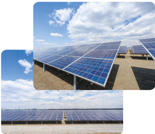
Solar panels (Solar Power Tomakomai Co., Ltd.)
