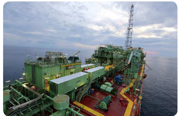
A floating production unit
