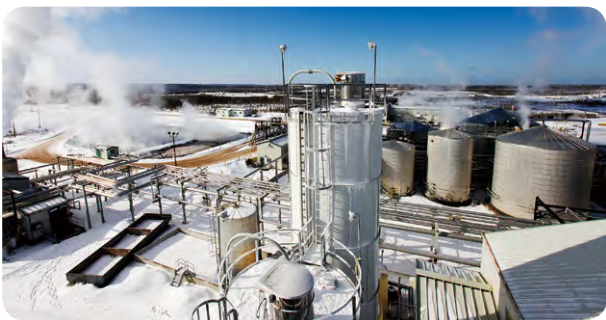
Canada oil sands production plant
