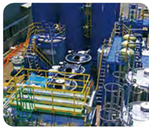
Pit-wastewater processing system
