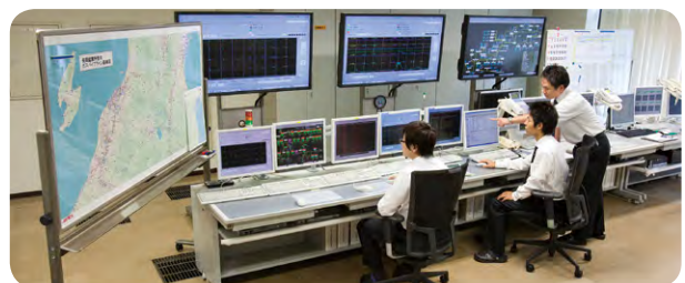
Nagaoka Pipeline Monitoring Center
