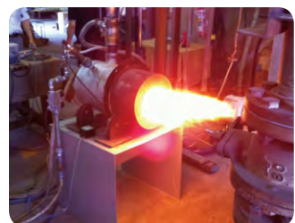
Wood powder boiler
