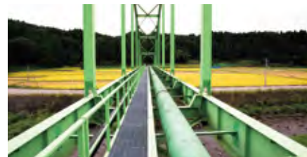
Niigata-Sendai Gas Pipeline
