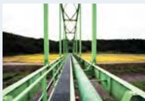
Niigata-Sendai Gas Pipeline
