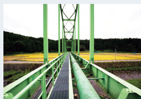
Niigata-Sendai Gas Pipeline
